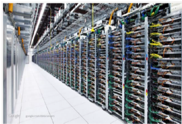
Racks of servers (and switches at the top), at Google's Mayes County, Oklahoma data center
